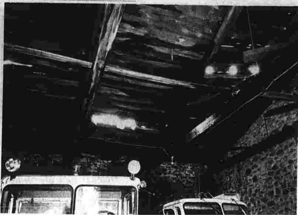
"Raindrops keep falling on my head" — So does snow, sleet, ice and sometimes sunshine at Coventry's town garage. Town officials say new facilities are needed; they're proposing to relocate the garage facility to a 22-acre site on Rt. 31 and Talcott Hill Rd. (Herald photo by Pinto)
